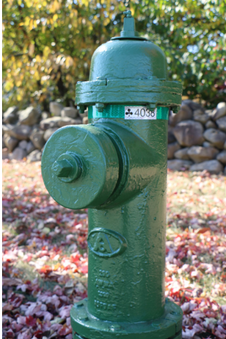
Green hydrants are City-owned.
