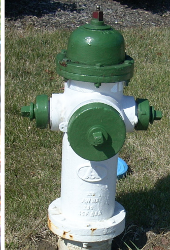
Green and white hydrants are privately-owned.
