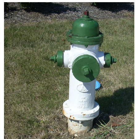
Hydrants with white bases are privately owned and are therefore not serviced by the City or the Fire Department.
